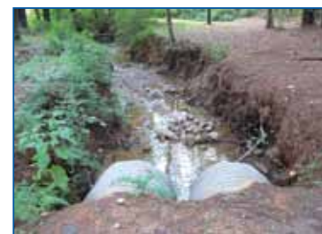
View of culvert outfall and associated scour hole prior to restoration.
